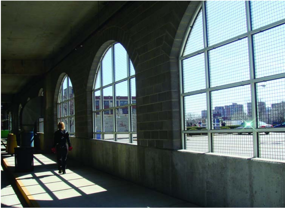
THE METAL SCREENS over the ground-floor windows at this Louisville, Kentucky, parking garage allow for natural surveillance while also preventing unauthorized access. Such screening also increases the likelihood that calls for help will be heard.
